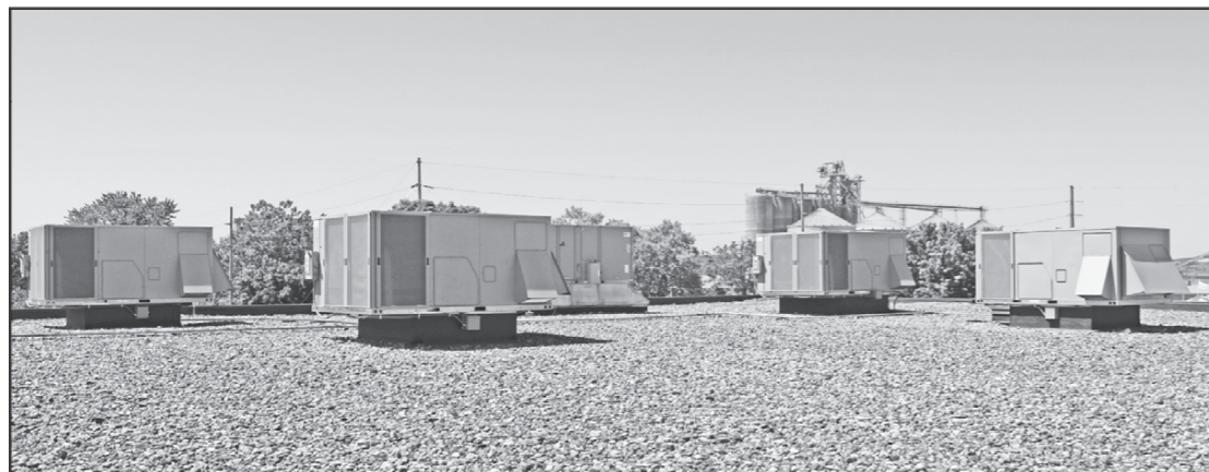
The YMCA's new HVAC system was installed earlier in June. (Photo submitted)
