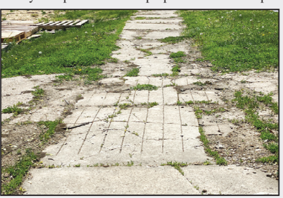
The sidewalk program being spearheaded by nuisance and animal control officer Bill Dietering would provide funding to Red Oak residents to repair damaged sidewalks such as these in the area of Reed Street. (Nick Johansen/The Red Oak Express)
